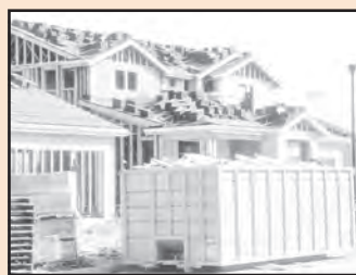
Debris Box Services
